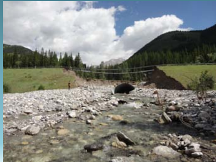
Hwy. 40 Lineham Creek – Washout of 4.3m SPE – 2013 Flood Event - Outlet
