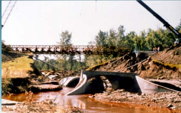
Culvert outlet after high water.
