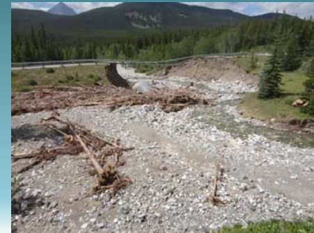
Hwy. 40 Lineham Creek – Washout of 4.3m SPE – 2013 Flood Event - Inlet
